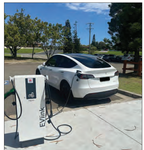
EV charger in Bermagui
