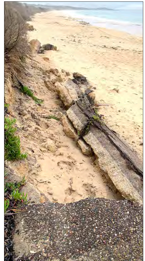
Erosion. Photo credit Sandra Renew
