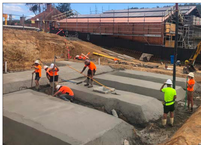
The Monarch building team at work completing the footings and under-slab waterproofing at the rear of the Village Square site in January.
