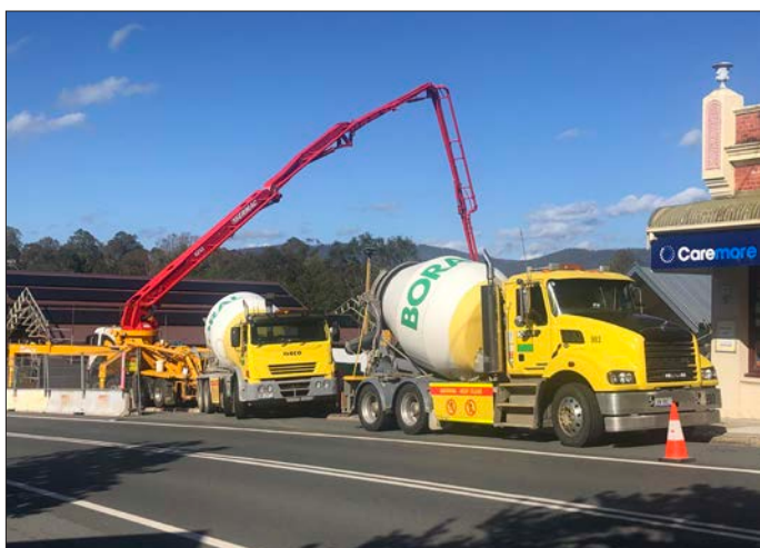
Concrete trucks and pumper delivering bulk concrete to the Village Square site in mid-January as the Rebuild Cobargo project fired up after a brief Christmas/New Year break.
