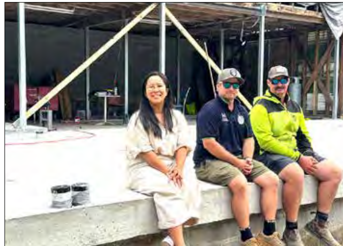
On the new slab - Steph, project manager, Hahn, the builder, and Tim, the site foreman.
