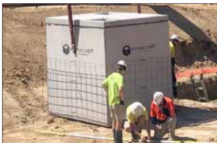
One of the large underground stormwater retention tanks being installed last month
