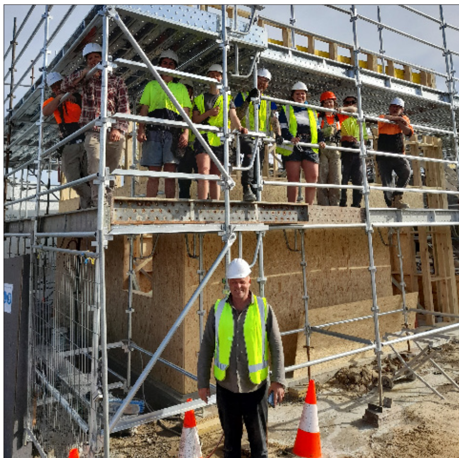
Jason Miles with his team at the Cobargo Resilience Centre. Up, up and away! The build is well under way.
