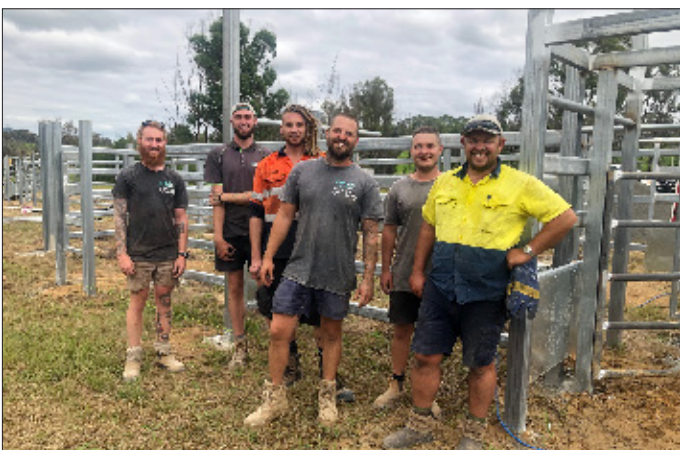
Tim Dummett and the ProScape Solutions team with carpenter, Luke Hoskins, working onsite at restoring the Quaama Sportsground
