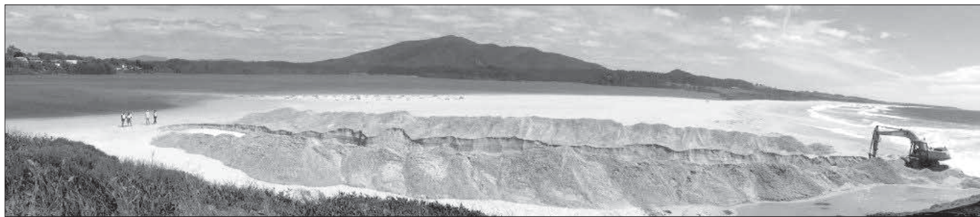
A panoramic view of the trench being dug to connect the lake with the sea (photo courtesy Kryisia St Clair)
